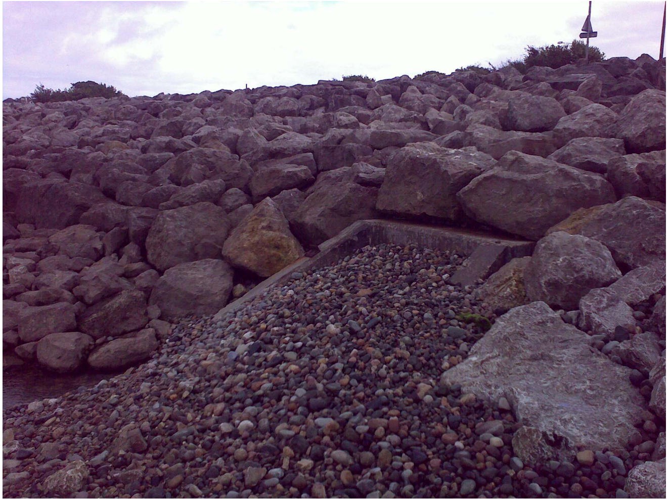
Outfall when blocked with 8 tonnes of shingle after a spring/ rough high tide.
